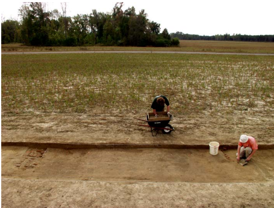
Plate 26. Test Trench 2000 at 31BR245 showing sections of brick foundations for east and west walls of a major structure, facing south.
