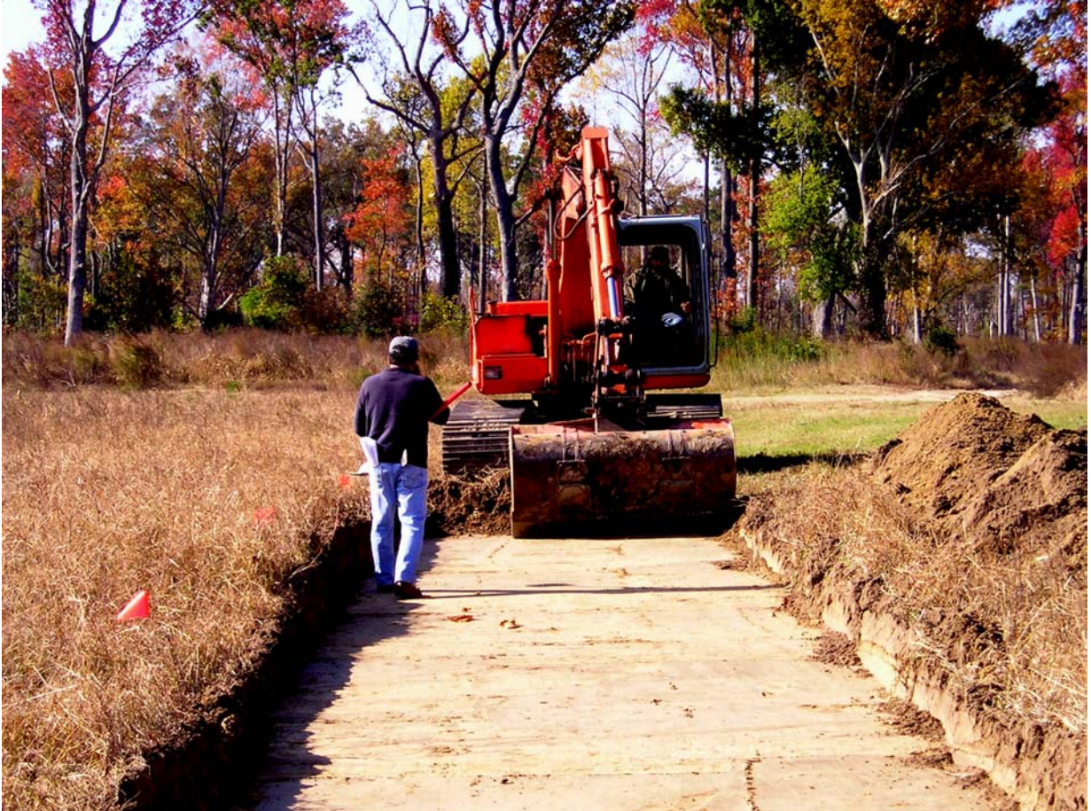
Plate 14. Mechanical cutting of test trenches at 31BR189 using an excavator with a smooth edged bucket.
