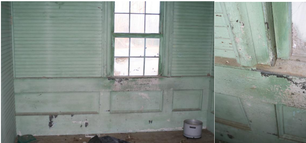
Figure 56: William Smithwick House, interior of dining building and detail of window molding and wainscoting.
