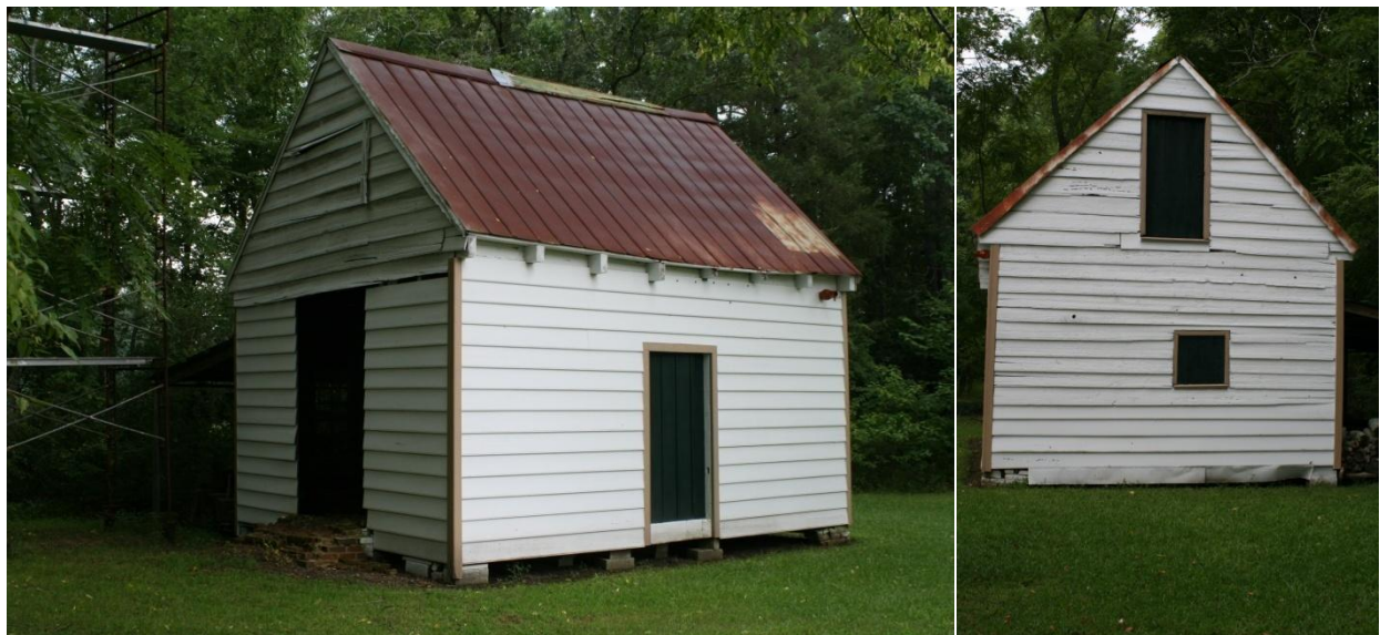
Figure 76 and Figure 77: King-Freeman-Speight kitchen, ca. 1810-1820. Note shuttered window opening and loft door.
