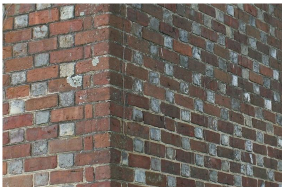
Figure 3: Detail of Jordan House brickwork showing handmade bricks with glazed headers laid in Flemish bond.
