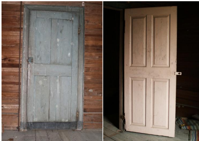
Figure 33: Asa Phelps House, flat and raised sides of four panel door with original light blue paint and dark gray-blue base which would have corresponded with a mop board of the same color.
