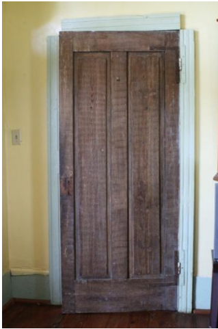
Figure 67: Sessoms House, ca. 1850-1860, two-panel door with faux graining and H-L hinges. Note that corner blocks are missing from fluted Greek Revival door surround.
