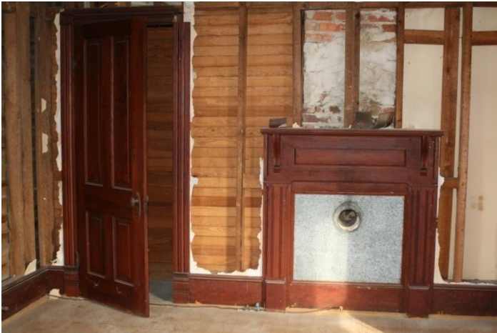
Figure 164: Eastbrook, second floor interior showing factory made mantel, door, and trim. Note that baseboard continues across the fireplace, which is fitted with a stovepipe.
