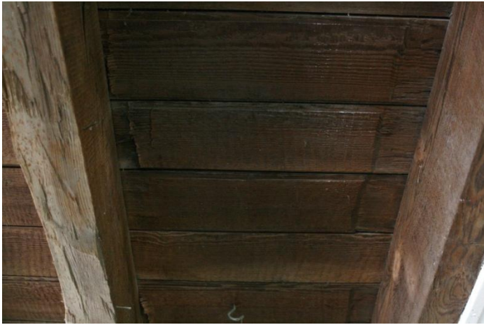
Figure 13: Sessoms House, ca. 1850-1860, underside of gauged and undercut floor boards, and hewn and sawn joists.
