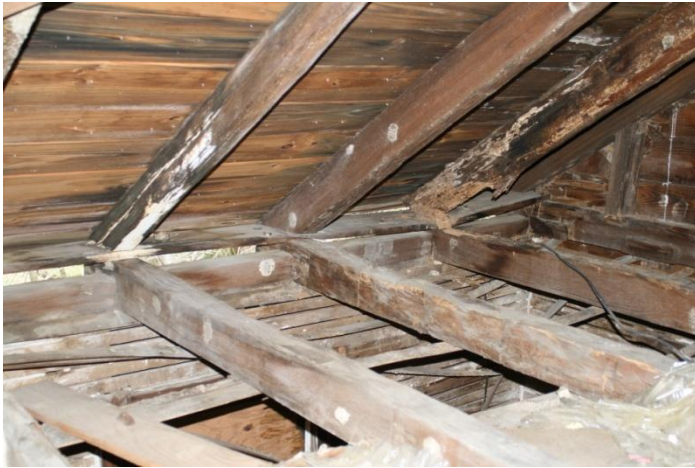
Figure 7: Asa Phelps House, board false plate at junction of rafters and ceiling joists.
