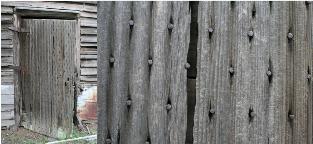
Figure 90 and Figure 91: Bond Haste smokehouse board-and-batten door and detail of wrought nails.
