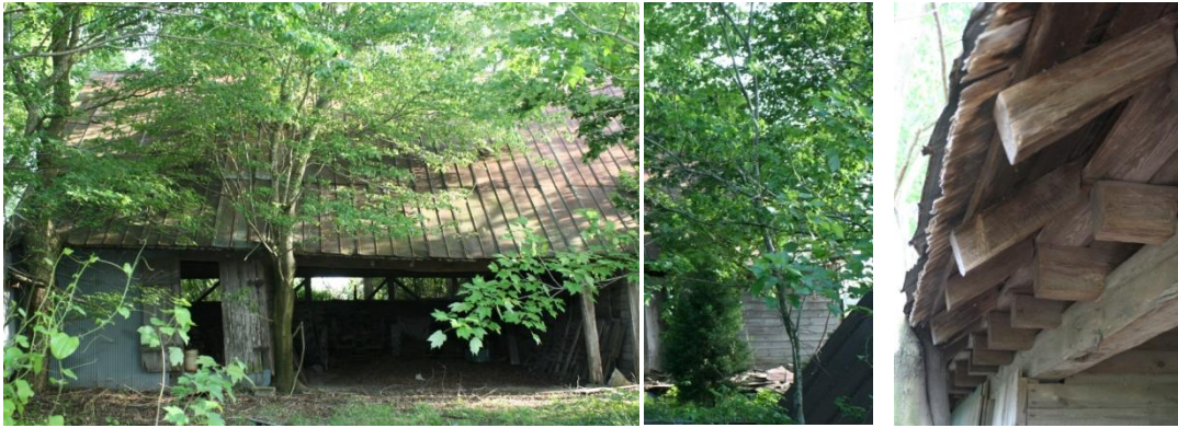
Figure 107: Henry House, ca. 1850-1860 cotton gin. Figure 108: Cotton gin plate, joist, false plate and rafter detail.
